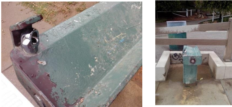
Figure 14 - Examples of poorly managed drinking fountains in Eagle Rock
