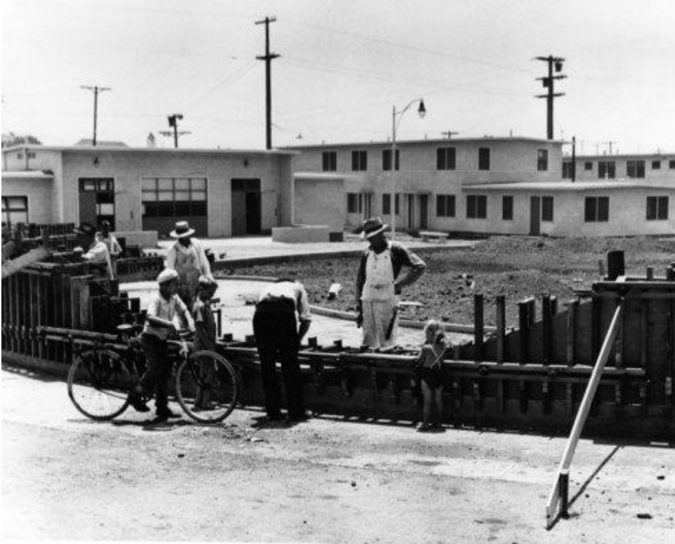
Figure 5. Greene, Jackie. Construction of Estrada Courts , Undated. Photograph. Los Angeles Public Library. Los Angeles. https://www.laconservancy.org/locations/estrada-courts .
